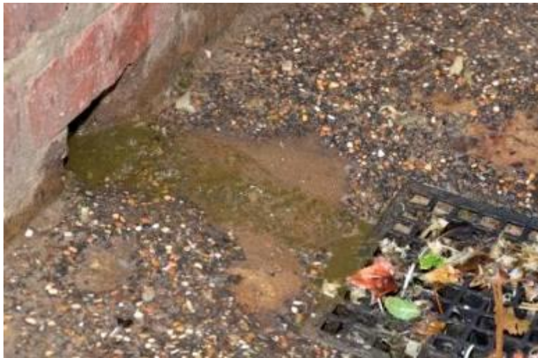
Do not allow run-off to contaminate walkways
