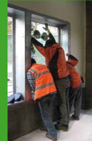
The windows in the new playroom are 40mm thick and very heavy!
