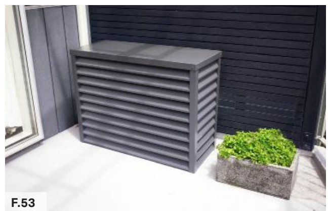
Figure 53: Air source heat pump housing covers the unit and harmonises with the building aesthetic
