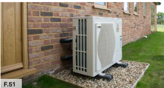
Figure 51: Air source heat pump unit
