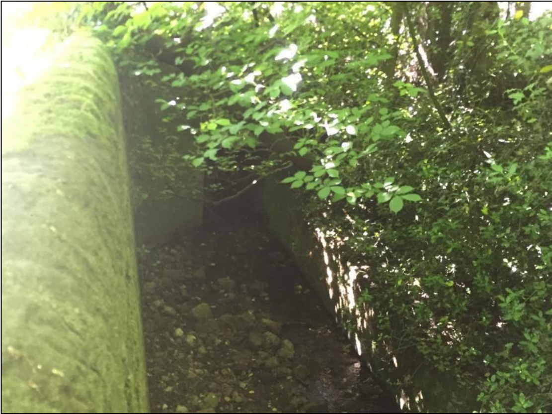
Figure B-5: Inlet to Church Bridge (looking downstream), where the headwall appears to trap sediment along the left hand bank
