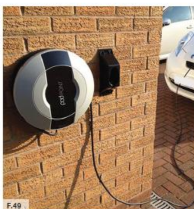
Figure 49: Home electric vehicles charging point
