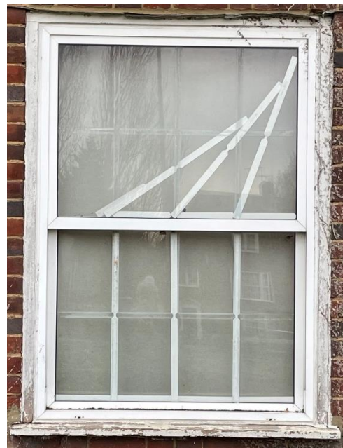
Figure 8: A rather unconvincing sash window where the sandwiched glazing bars have failed.
