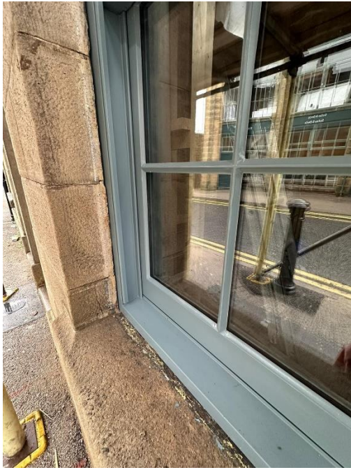
Figure 3: Newly installed slim double glazed Accoya timber sashes with through glazing bars. These replaced white uPVC casements in a non-designated heritage asset.
