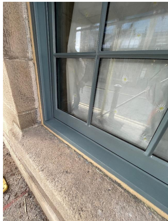
Figure 16: Burnt sand mastic pointing to seal around the timber frame in a buff stone colour.
