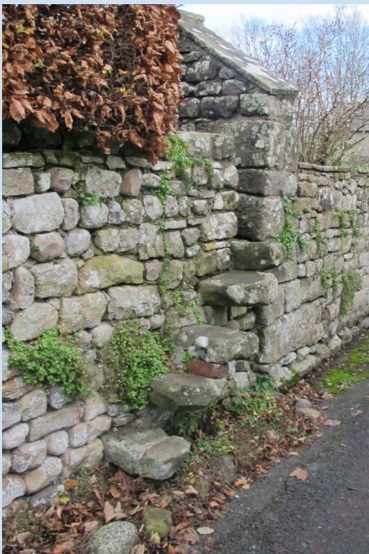
Fig. 12 Traditional drystone boundary walls characterise the village of Arkholme, some with flat coping stones.
