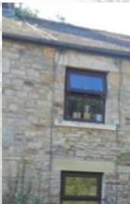
Fig. 30 Inappropriate alteration to windows to a mock sash style.
