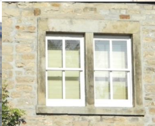
Fig. 31 Retention of traditional timber sliding sash windows contribute to the historic interest of the area.
