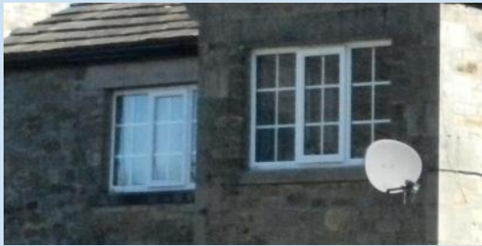
Fig. 20 Modern satellite dishes and PVCu windows negatively impact historic interest of parts of Melling's conservation area.
