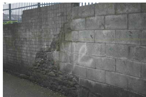
Inappropriate repairs on Church Walk
