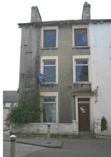
Run down and vacant property
