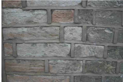
An example of bad pointing
