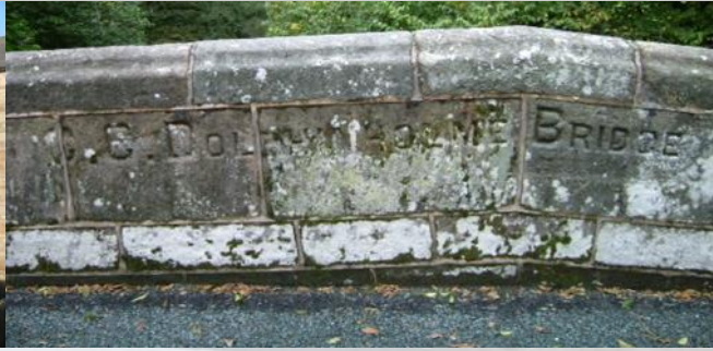
Fig. 18 Dolphinholme Bridge dated 1791 is constructed in sandstone ashlar with a segmental arch.
