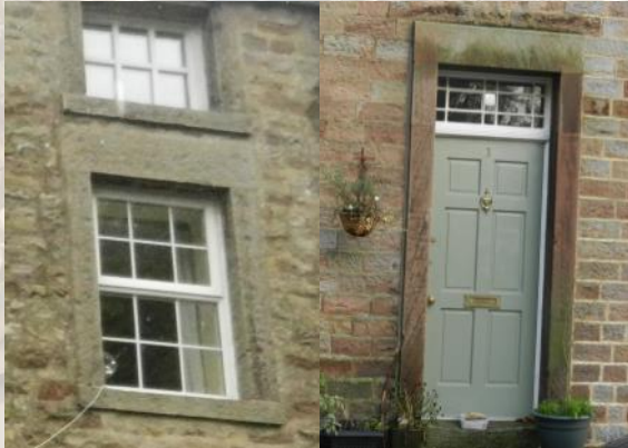
Fig. 34 Traditional sash windows have been replaced with modern upvc.
