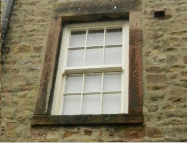
Fig. 10 Window at Corless Cottage is a traditional timber six-over-six paned sliding sash.
