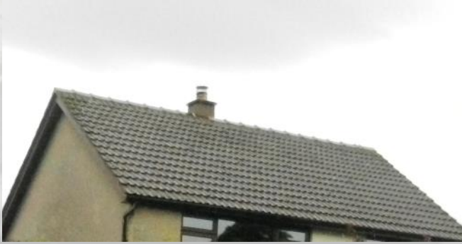
Fig. 26 Contemporary unnatural materials such as concrete pantiles for roofing.
